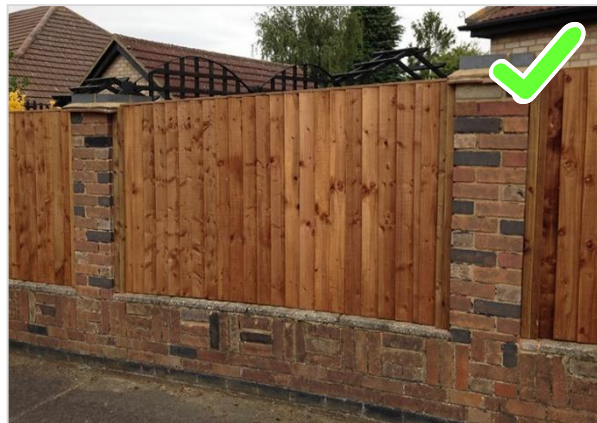
Close boarded fencing can be combined with walls and pillars of an appropriate style and materials to provide a more acceptable boundary treatment (subject to appropriate wildlife connectivity measures)
